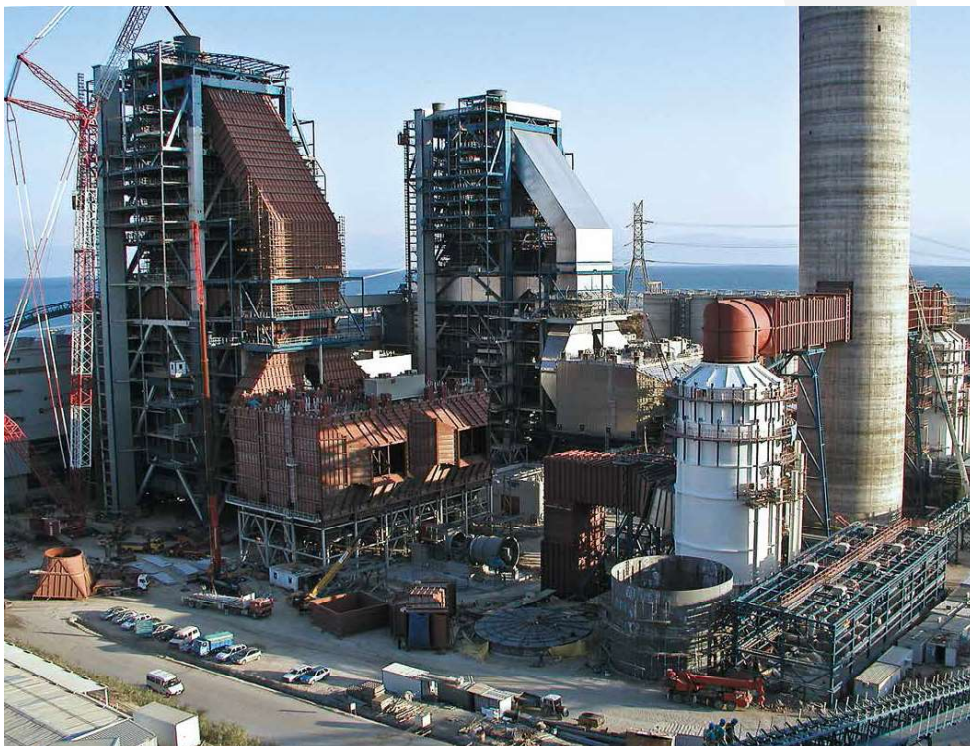
Construction of coal fired power plant in Turkey ditec supply of rubber and fabric expansion joints
