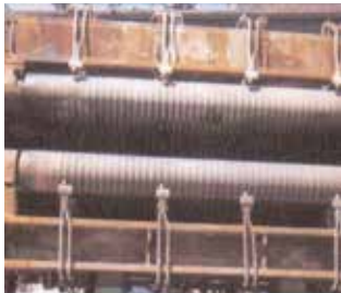
Air-mist nozzles fed and installed by means of small and long hydraulic pipes
